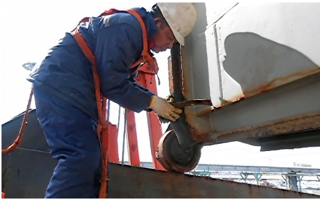
Figure 32 (a and b): Maintenance of rubber packing
