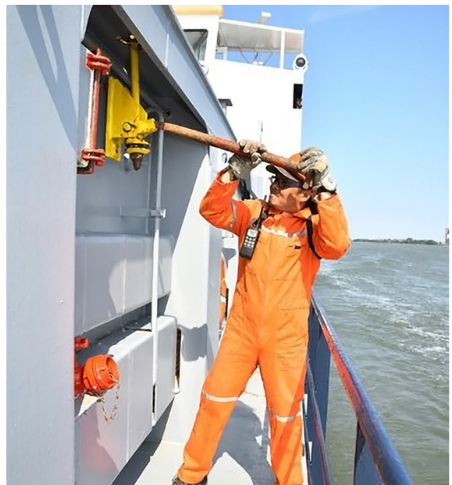
Figure 39 (a and b): Maintenance of hatch cleats
