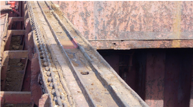
Figure 37: Poorly maintained drain channel
