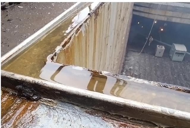
Figure 13: Blocked drain channel
