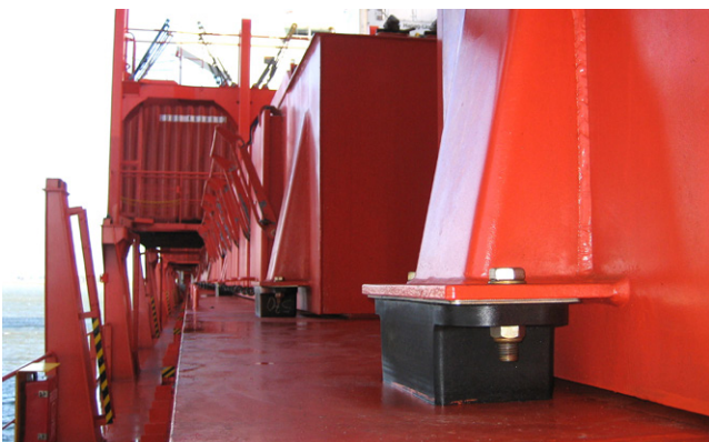
Figure 22: Landing pads – check if they are worn down
